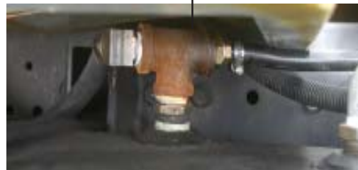
Fuel Lines From Tank
